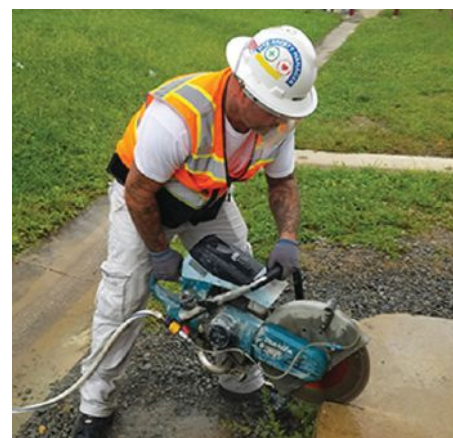
Applying water to a saw blade when cutting materials that contain crystalline silica — such as stone, rock, concrete, brick and block — substantially reduces the amount of dust created during these operations.
